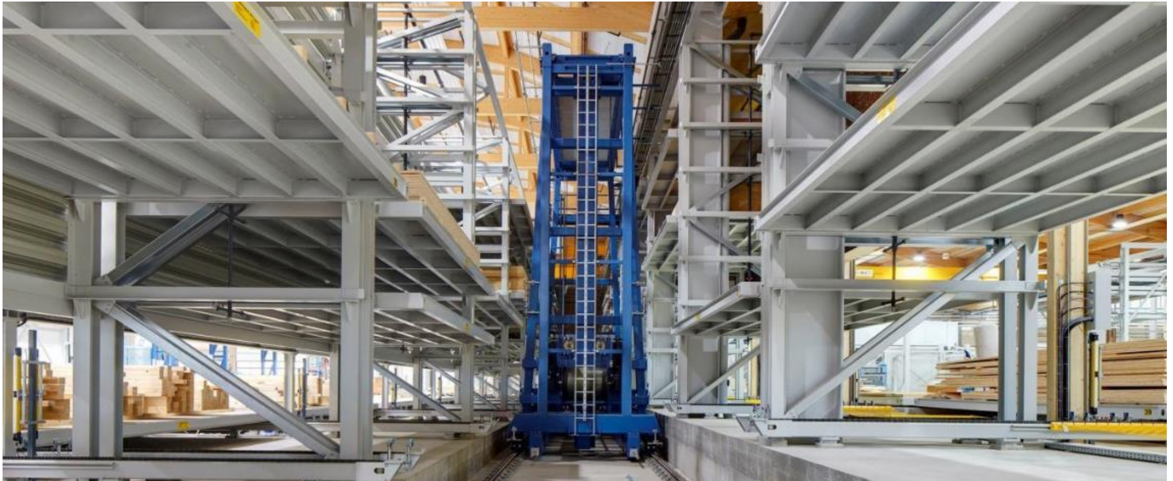
Shelf access equipment with storage and retrieval conveyor for various materials and elements at Renggli
